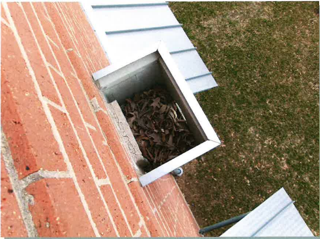
Debris filled conductor head.
