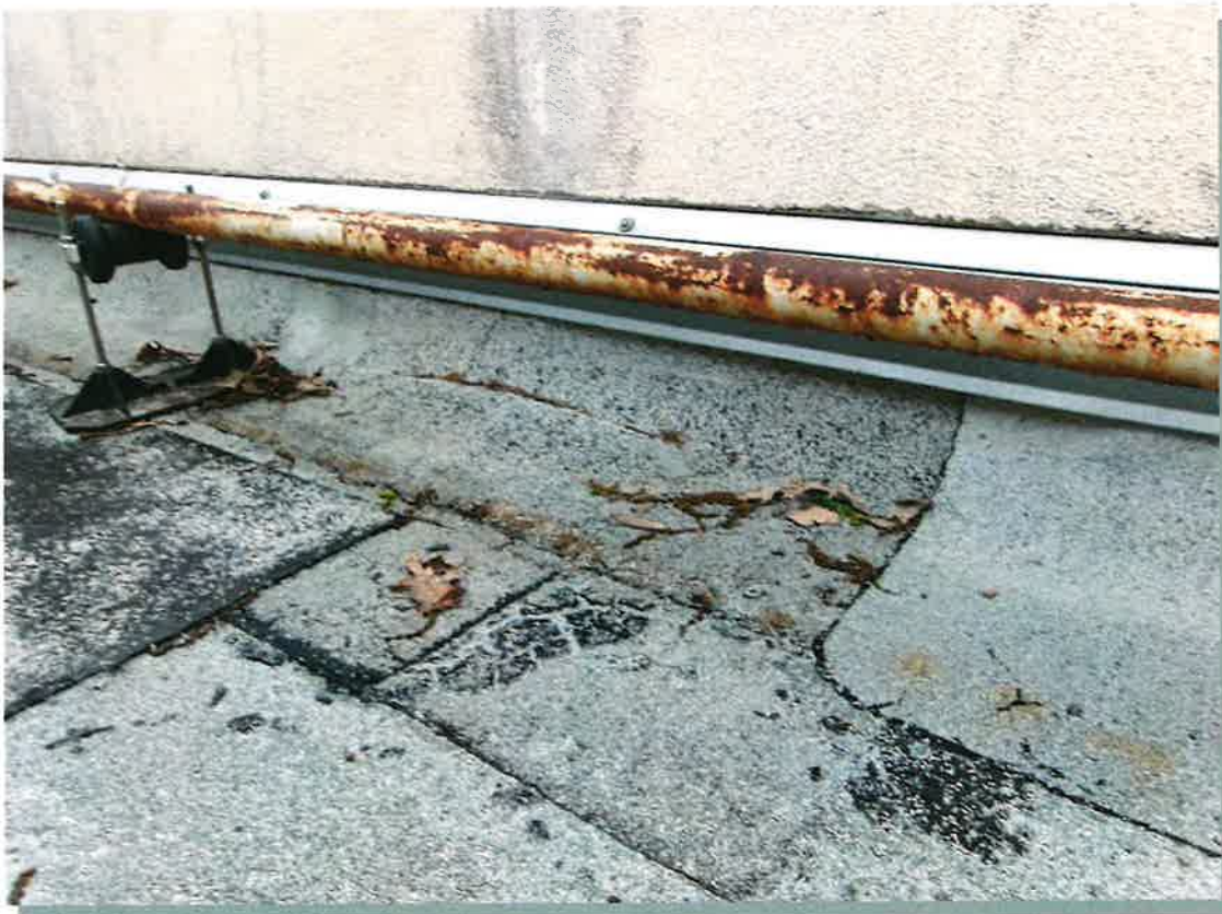
Blister development along perimeter wall flashing.
