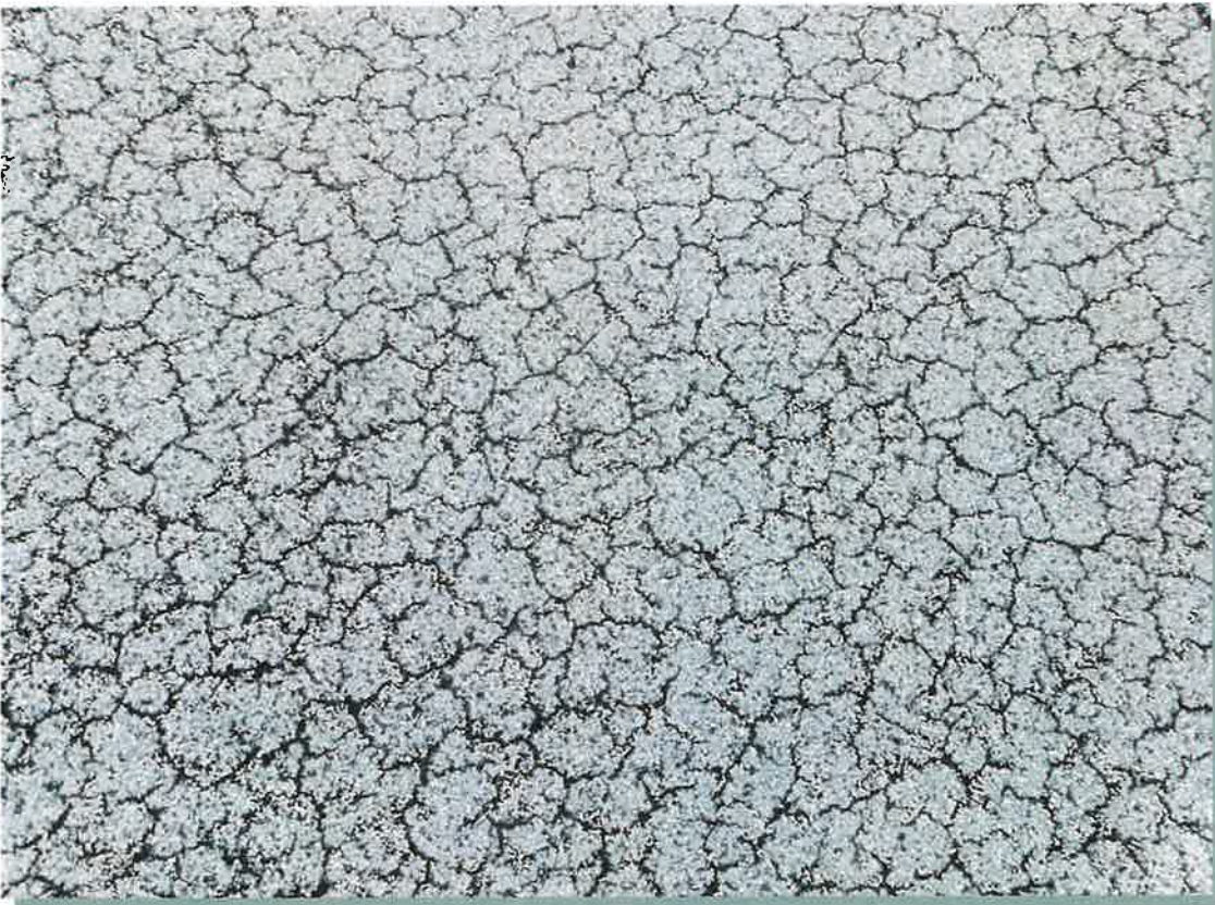
Membrane cracking in field of roof.
