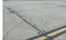
D Cracking - Example 2
