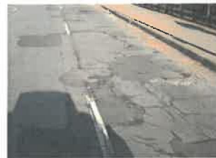
Sample Poor to Very Poor segment (25-40)
