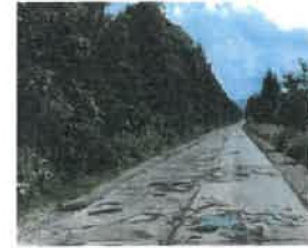
Sample Very Poor to Failed segment (0-25)
