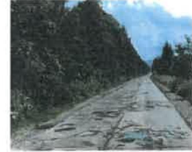
Sample Very Poor to Failed segment (0-25)
