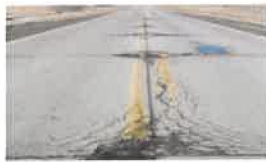
D Cracking - Example 1
