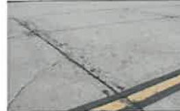
D Cracking - Example 2
