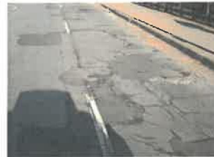
Sample Poor to Very Poor segment (25-40)
