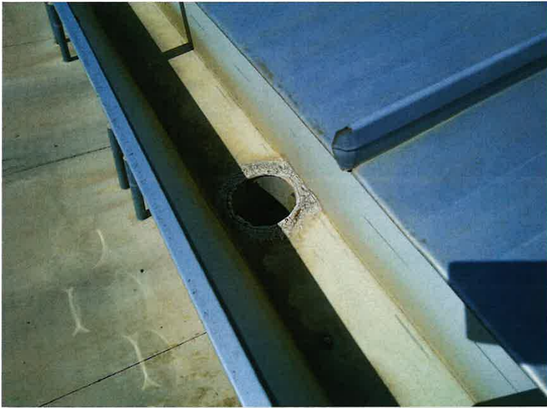
Sealant failure at downspout connection.
