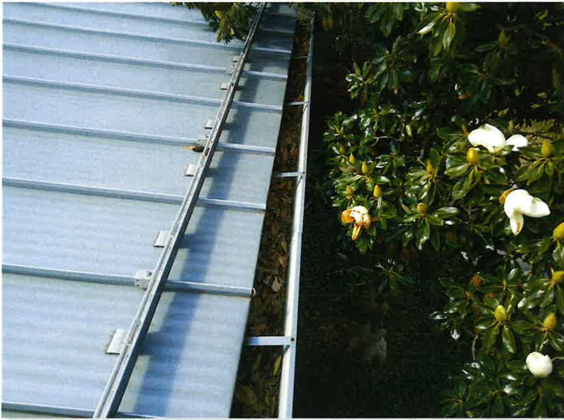
Leaf debris and gutter.
