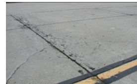
D Cracking - Example 2
