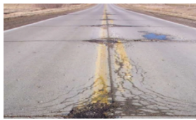
D Cracking - Example 1
