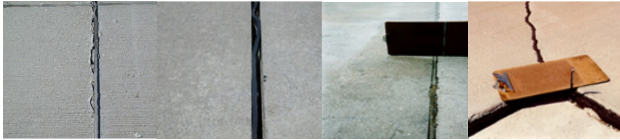
Joint Seal Damage - Example 1
